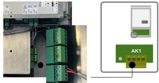
Figure 14: AK1 cable connection.
