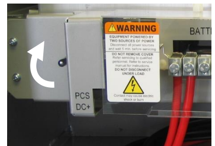
Figure 14: Battery breaker disconnect turn ON.
